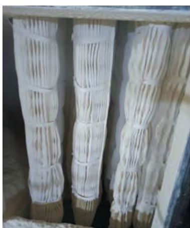
Fig. 6. Bag filter after modernization
